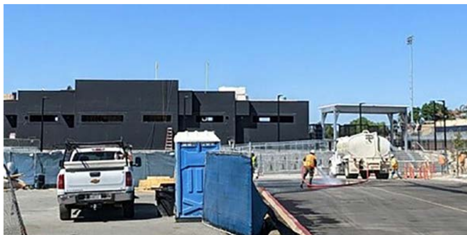
By Sept. 22, this is the current progress of the front side of the stadium entrance in front of the schools parking lot. There are construction workers building more over Fall Break. PHOTO TAKEN BY NICO GATTEN
